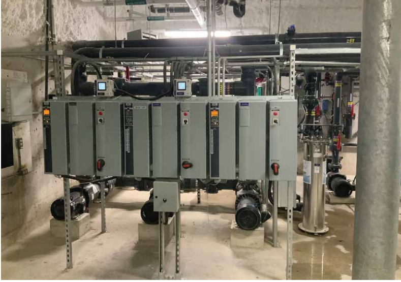
The upgraded mechanical systems at the revamped Kidstown Water Park in Scarborough, Ont., has offered the operator greater control.
